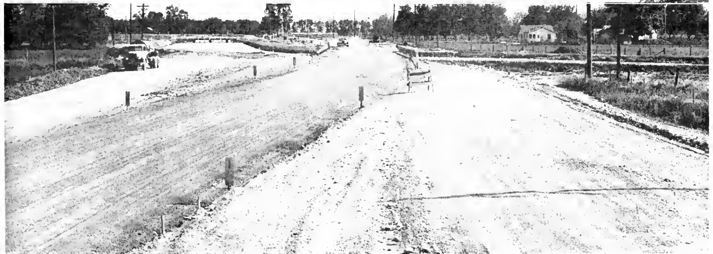
UPPER—View of project south of Gustine, looking north toward Borelli's Corner, showing new bridge with new alignment curving to right. CENTER—Bridge of Gustine Canal. View looking westerly showing bank lining. LOWER—View of project south of Gustine looking south, showing new alignment of south connection.
